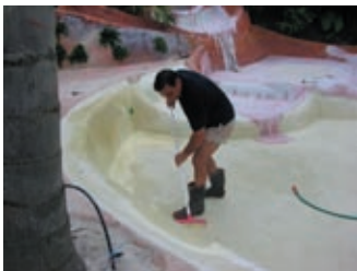
Hard at work: Dave does some acid etching, the last step before the pool is filled.
